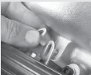
305. If you're running the taller injectors, the 0.500" tall spacers from the Katech adapter kit are placed between the fuel rail brackets and the manifold. Note that the long slot side of the fuel rail brackets must be placed at the manifold bosses.
