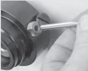
200. Next, the hole is reamed to 3/16", using the kit's reamer on an electric drill, in a single pass.
